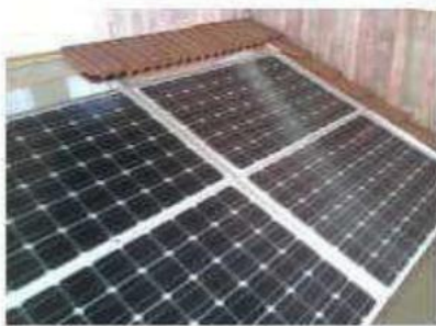
Installation photovoltaïque raccordée
